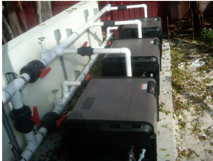
Main Pool – Heater
